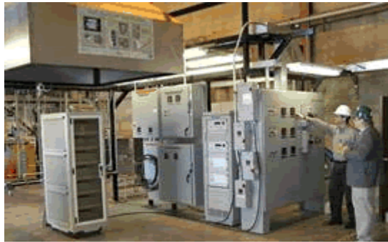
Fuel Cell Test Facility
