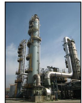
CO 2 capture Plant (450 t/d)
